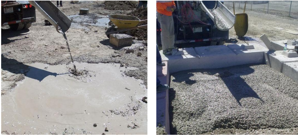
Figure 3: Slag and RCA mix (left) cement &RCA mix (right). Note that the excessive water in the slag mix is attributable to the presence of water in the trench prior to placement of the U-fill mix
