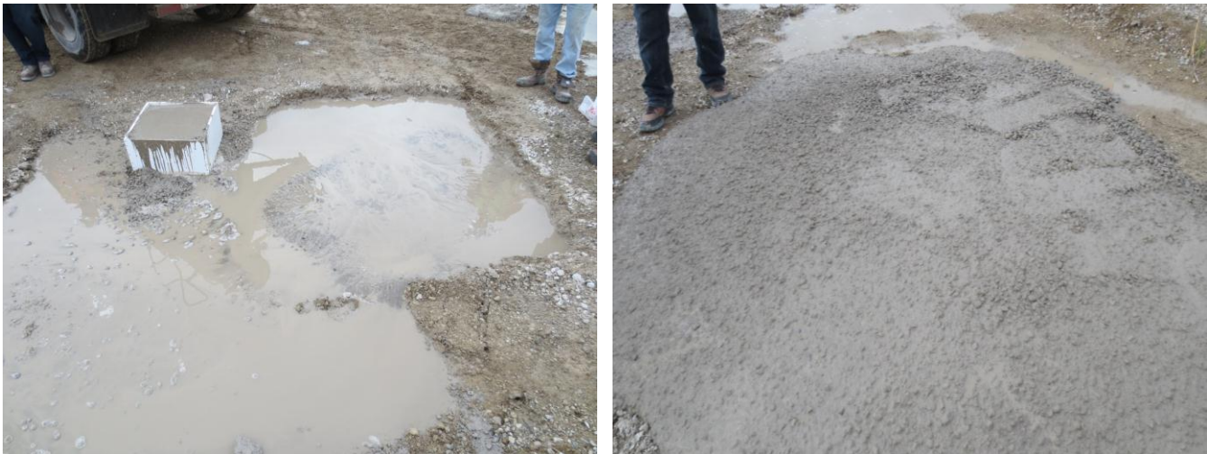
Figure 4: Field trial mix containing 50% Gravel, 30% RCA & 20% Sand (Left) & Field trial mix containing 70% Gravel, 30% RCA & 20% Sand (Right)
