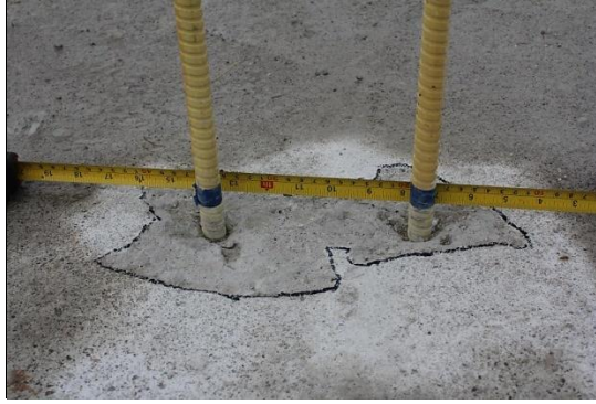
Figure 3. Sample of mode of failures observed in specimen D-N5-150S-S3
