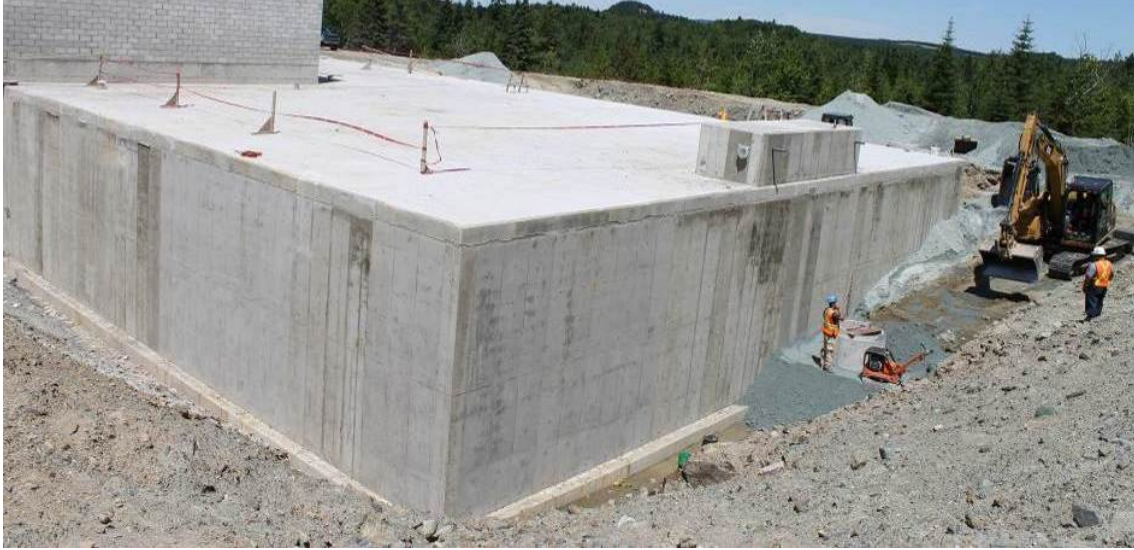
Figure 7: Overview of the completed tank through the leakage test and prior to backfilling
