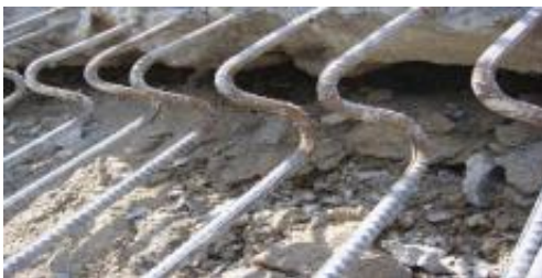
a) Separation in Concrete Face of Zipingpu in China (Chen and Han, 2009)
