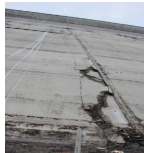
b) Dame of concrete slabs along joints of Zipingpu CFRD in China (Chen and Han, 2009)
