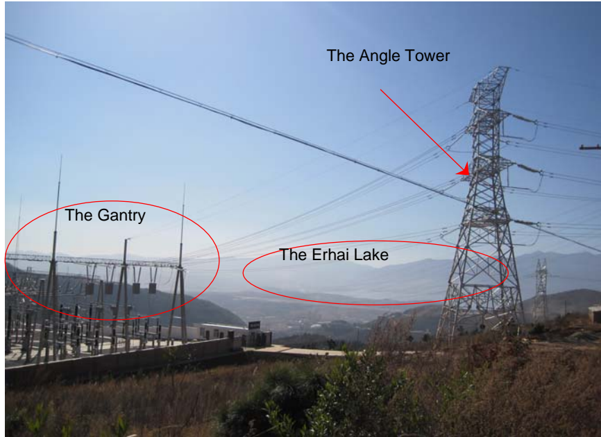
Figure 2: 220-kV Haidong Transformer Station
