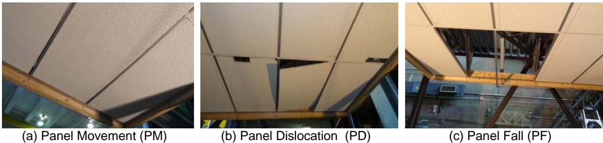
Figure 6 Failure modes of the acoustic panels
