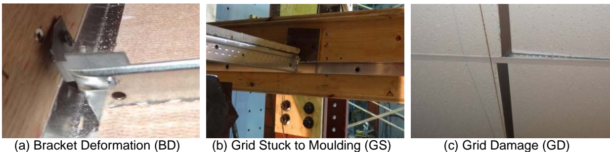
Figure 7 Damage patterns of the suspension grid system
